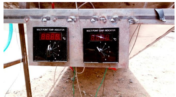
Fig.6 Temperature indicators for measuring HTF and PCM temperatures.
