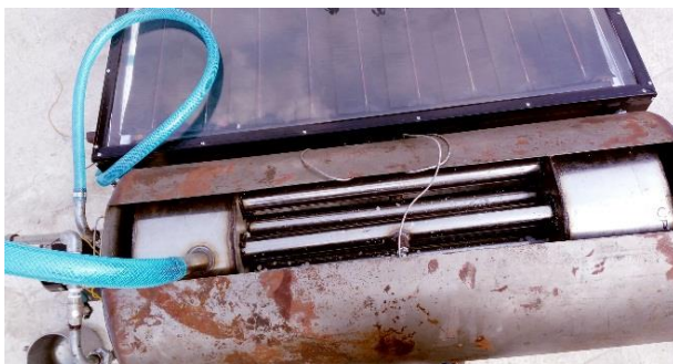
Fig.5 Inner view of TES tank
