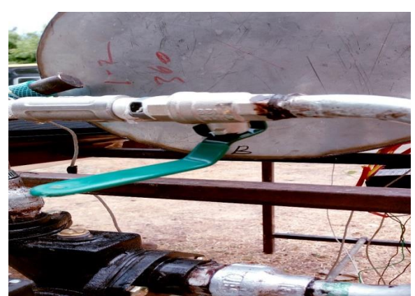
Fig.8 Flow control valve
