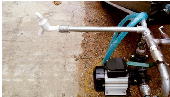
Fig.9 Tap for extracting hot water and pump for water circulation.
