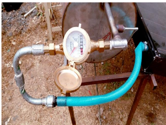
Fig.7 Flow meter to measure the rate of flow of HTF.
